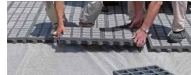
For a more efficient procedure, the TTE® elements can also be laid pre-filled as TTE® directPAVE. Mechanical installation is also possible in this way.
